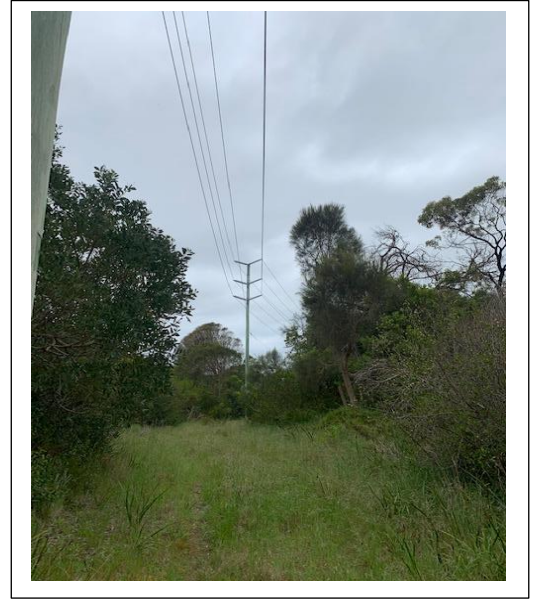
Location 2 Pole 161 Sheaok 3 Metres – Code 2024
