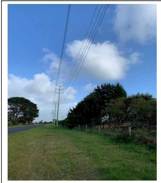
Location 1 Pole 51 Pine 4 Metres – Code 2024
